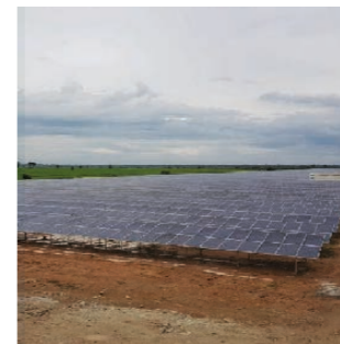
10.6 MW SOLAR FARM
