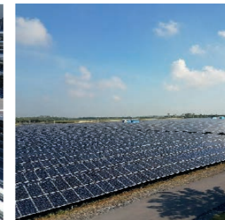
4 MW SOLAR FARM
